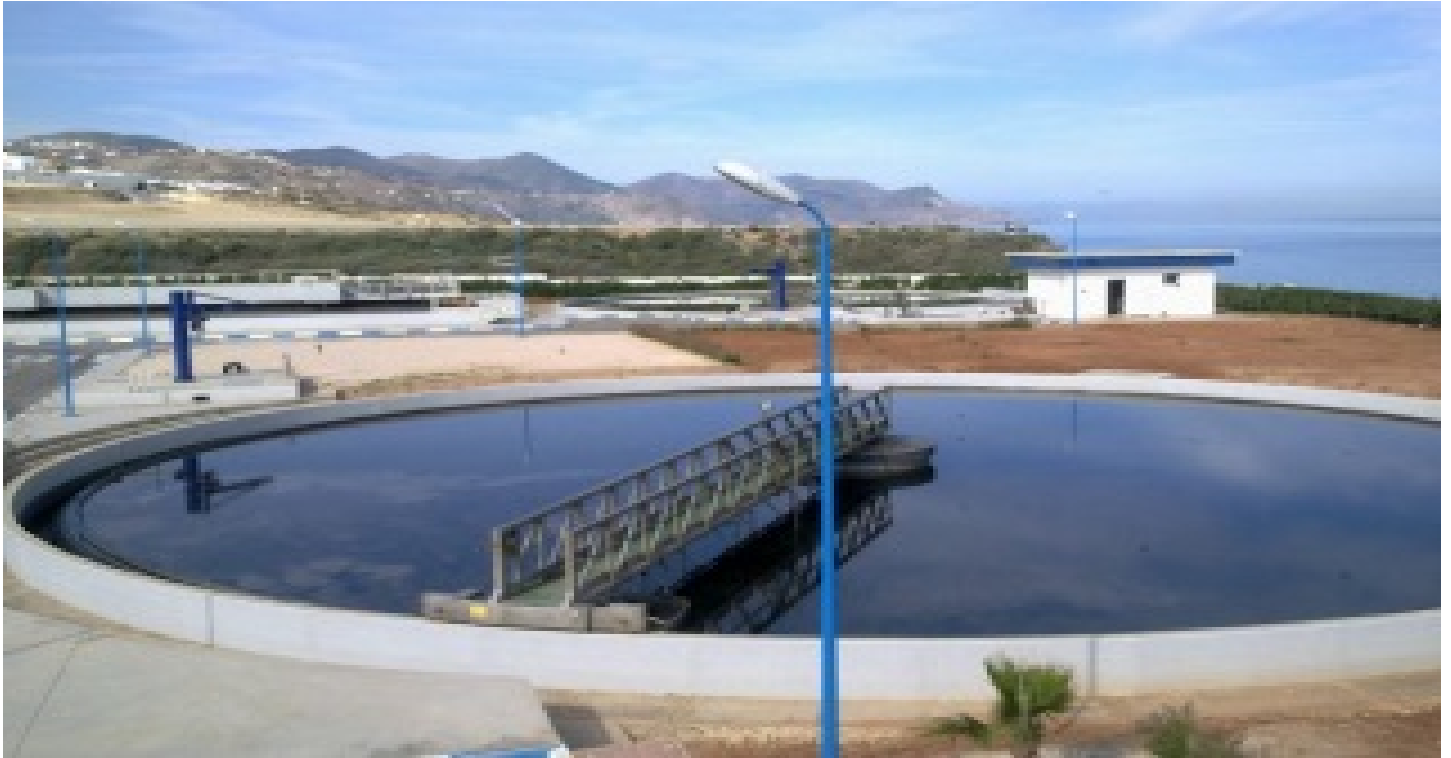
Effluent Treatment and WWTP Operation
